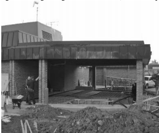
Fig. 5 GFRP reinforced concrete slab for MRI rooms in hospital (York, Maine)
