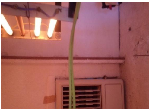
Figure 4. Heater on condition in room
